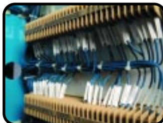
Precise wiring and labeling
